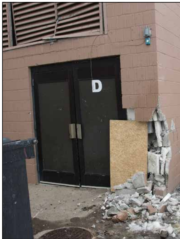
Damage to an outer wall of Pagosa Springs Middle School following an alleged drunk-driving incident Jan. 16. In the incident, a man is suspected to have eluded a sheriff's officer and driven the wrong way down a one-way street before crashing into a dumpster and the wall.
