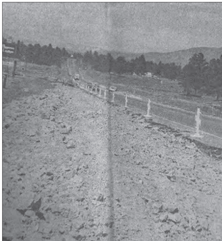
From the June 12, 1980, Pagosa SUN — WIDENING — An acceleration-deceleration lane is being added to the highway at Pagosa. This stretch is in front of the Pagosa Lodge. The work is being done by contract from Eaton International and the engineering is being done by the State Highway Department, who will also resurface the highway for a seven mile stretch, including the new project.
