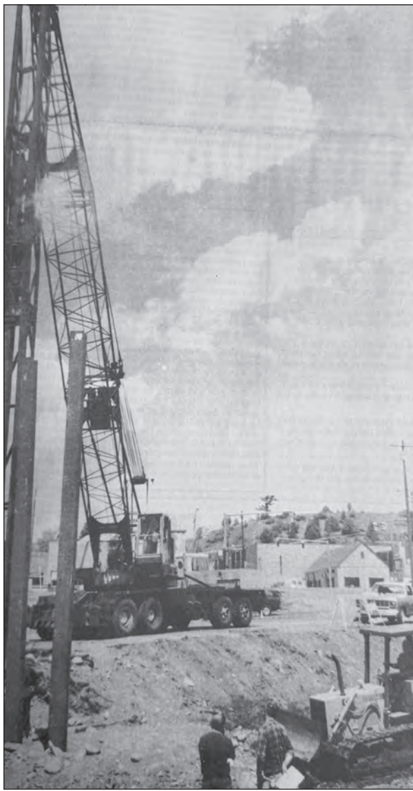
From the June 8, 1989, Pagosa SUN — The persistent pounding of this pile driver echoed through downtown Pagosa Springs last Thursday and Friday. The noise continued on Monday and Tuesday of this week as 40-foot steel I-beams were sunk on opposite sides of the San Juan River. G.A. Western Construction Co. of Grand Junction hopes to have the new bridge for the 4th Street/Light Plant Road crossing completed by the end of this summer.
