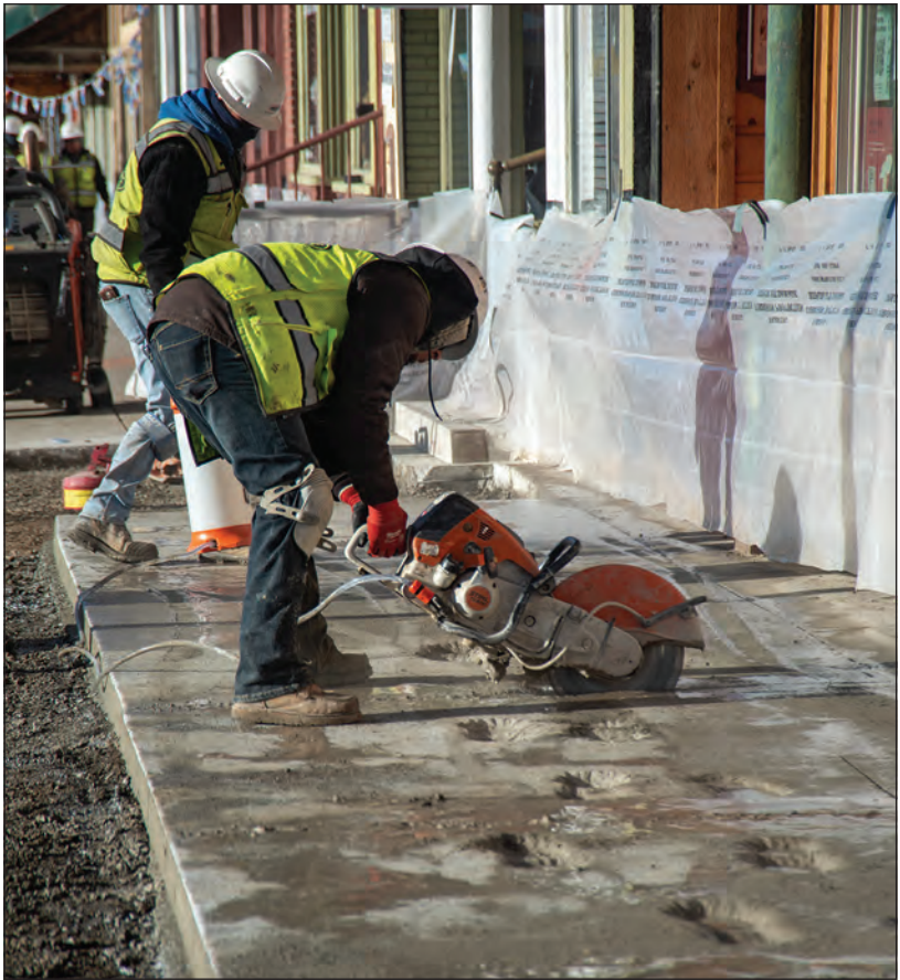
SUN photo/Randi Pierce U.S. 160 reconstruction personnel work prepping newly poured concrete for removal Wednesday morning after someone entered the work zone the night before and damaged the concrete.
