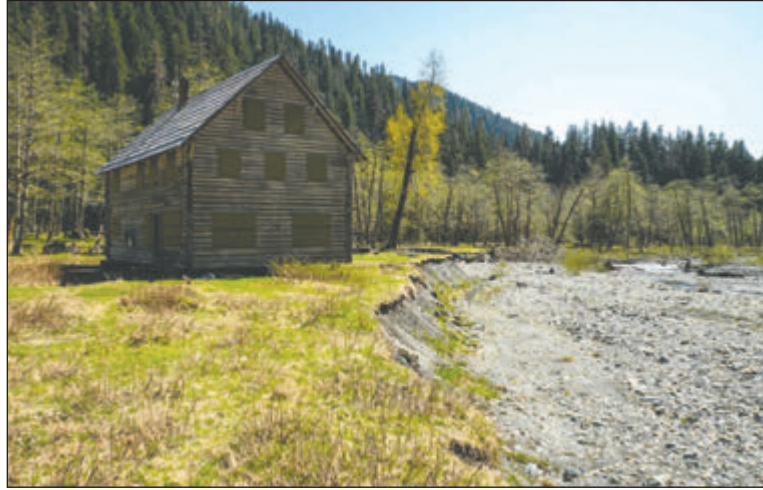
The historic Enchanted Valley Chalet sits precariously close to the encroaching riverbank. National Park Service photo
