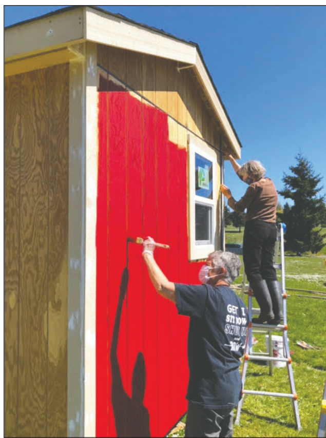
Volunteers from the Community Build Project joined efforts this year to construct a series of "wooden tents" that will be used by Bayside Housing and Services to provide transitional housing in the Eisenbeis Addition. Photo courtesy of Judy Alexander
