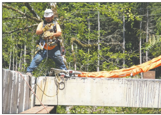
Slabs for the approaches to the temporary bridge are put into place Thursday. Leader photo by Brian Kelly
