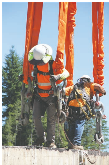
Straps are moved into place to help lift a slab into place for the temporary bypass bridge at Shine Creek. Leader photo by Brian Kelly
