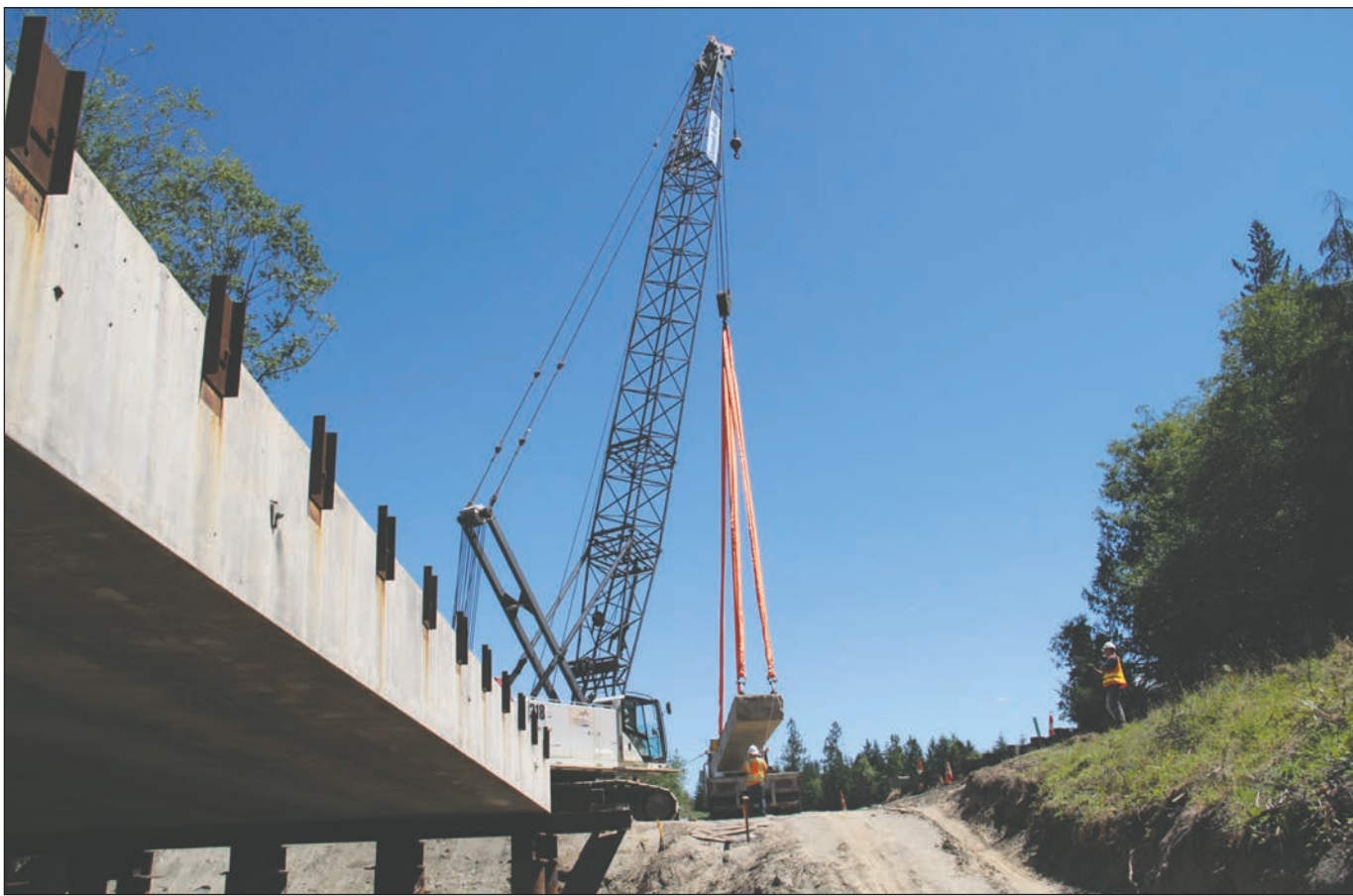
A crew with Seton Construction moves a concrete slab off a flatbed semi-trailer truck for use on a temporary bridge along Highway 104 west of Shine on Thursday. Leader photo by Brian Kelly
