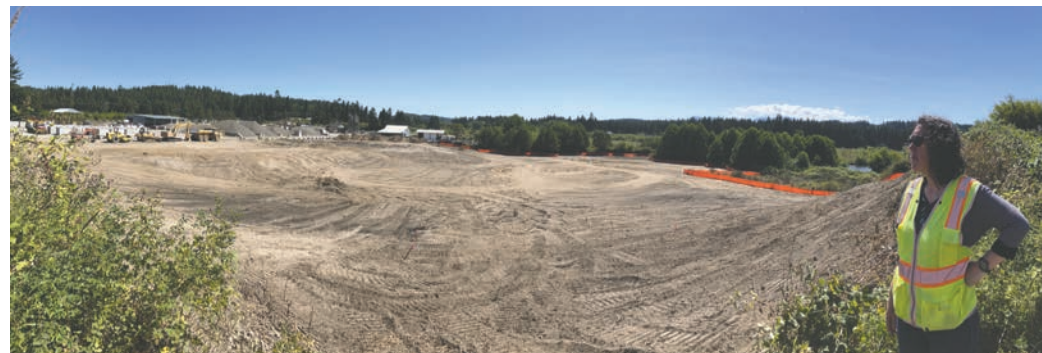
Wastewater Project Manager Samantha Harper surveys the construction site for the treatment and percolation pond that will be part of the new sewer system for Port Hadlock-Irondale. Photo courtesy of the Jefferson County Public Works Department
