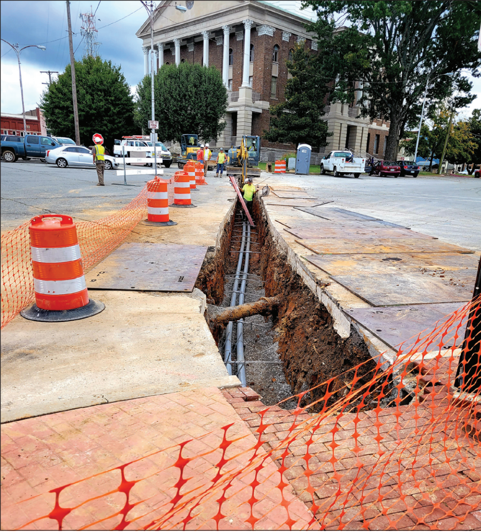
T-G Photos by Zoe Haggard The installation of underground electrical conduits at the corner of Holland and Spring streets is scheduled to be completed next Tuesday, according to Mike Clanton, one of the site's overseers. Completion for the square's entire underground installation is planned for next April.
