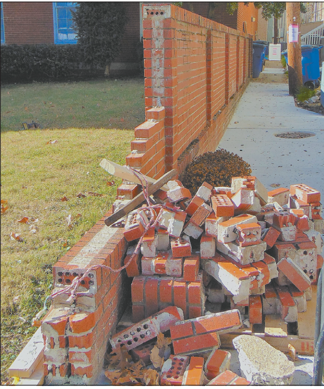
Oops... like living on a construction site, accidents are bound to happen—like when one of the workers backed some equipment into a 4-foot brick wall at Main & McGrew's alley way, knocking down a chunk of it.
