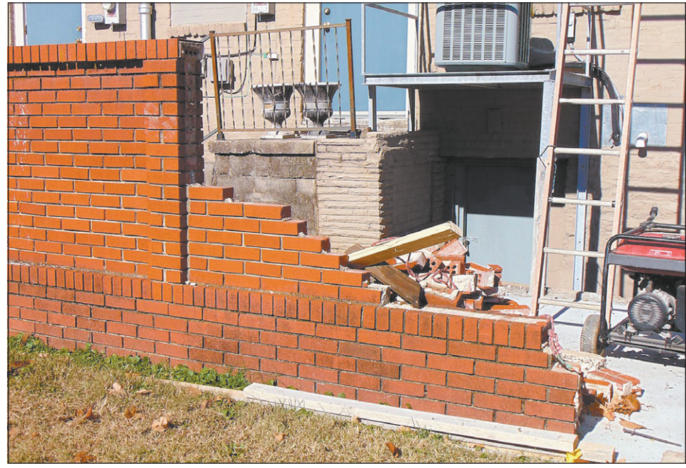
Danielle Armbruster, owner of The Shops at Main & McGrew on South Main right off the public square, said she isn't mad that this 4-foot wall by her antique store was demolished in the midst of City sidewalk construction. But it's been two months since the City told her it would be fixed.
