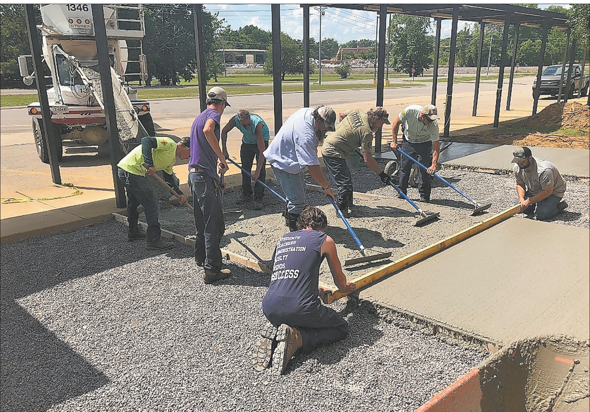
Bus riders at Shelbyville Central High School are going to have a new sidewalk next year, making it safer for students to load onto the buses. Maintenance crews here are pouring concrete for the new sidewalk.
