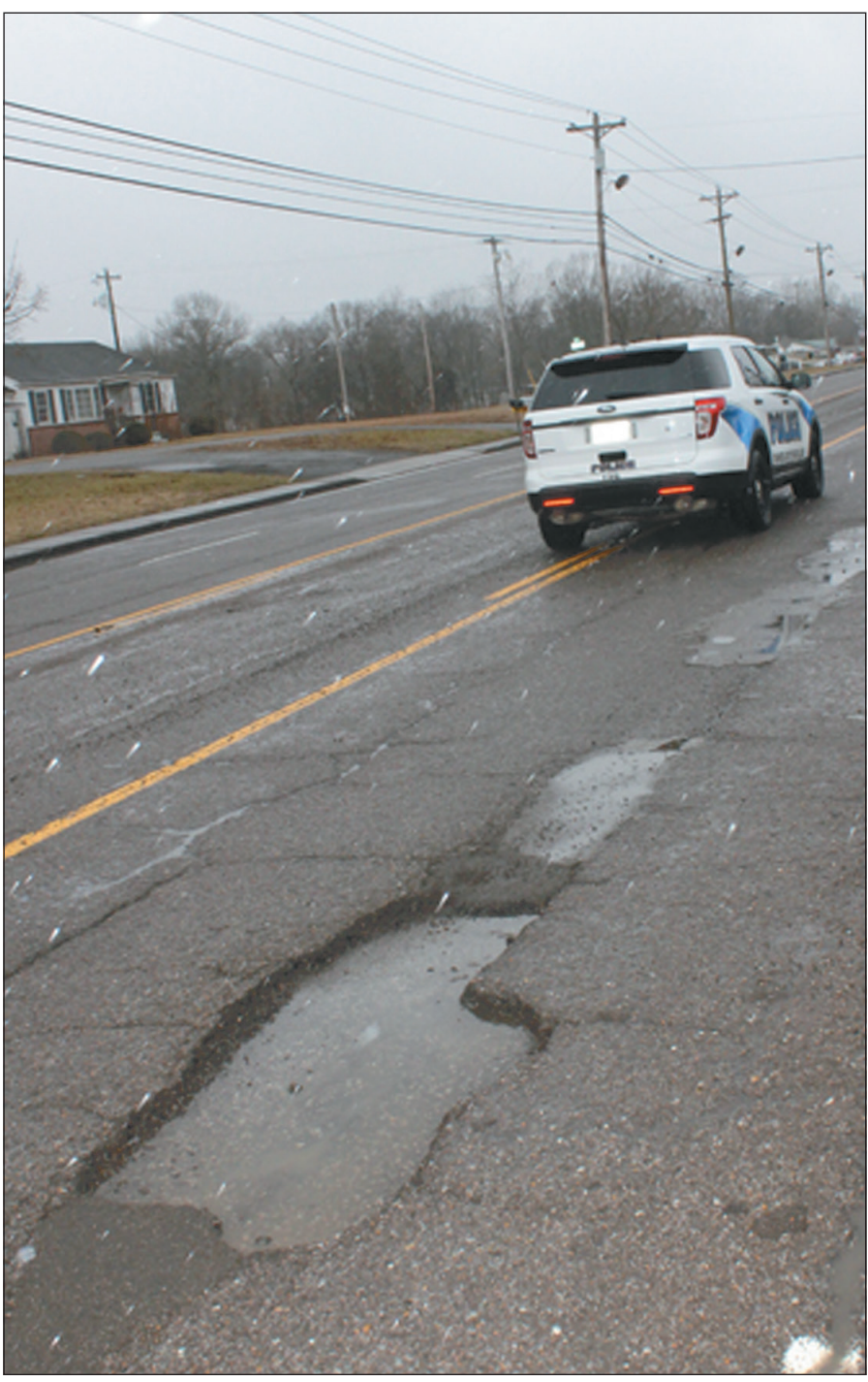
T-G Photo by David Melson A Shelbyville police officer swerves left to avoid large potholes on Madison Street near Learning Way Elementary School as snow falls Friday. The frequent winter rains interspersed with below-freezing spells are wreaking havoc on roadways across Shelbyville and Bedford County. Some of the holes are clearly large enough to cause alignment damage to vehicles.
