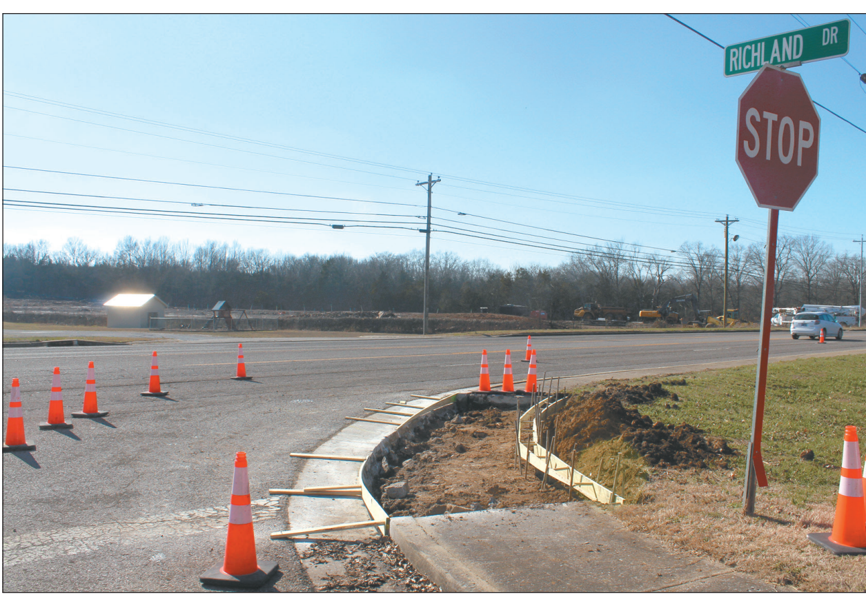
PROGRESS IN ACTION Sidewalks are being rebuilt along eastern portions of Madison, including at the intersection of Richland Drive. Across the street, construction is in progress on an unrelated new housing development.
