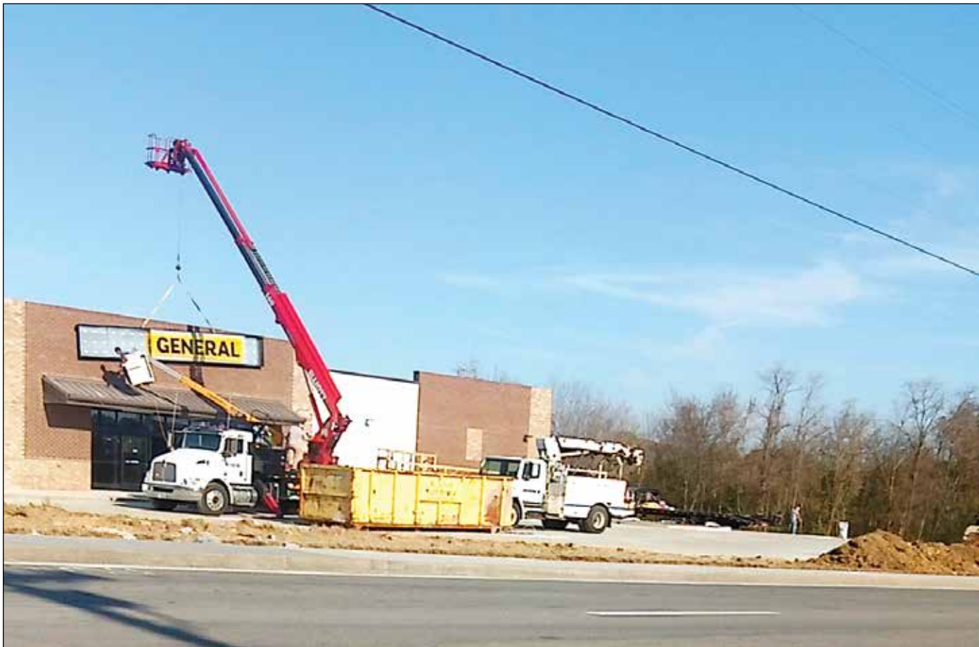
ANOTHER DG - Workers hoisted the official sign to the front of the newest Dollar General in Bedford County on Monday. There are at least nine now, located throughout Bedford County. This one is located off Madison Street, near the 41A South and Wartrace Pike intersection.
