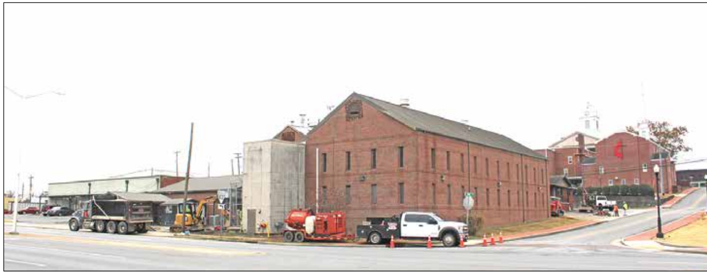
The county jail of the 1980s is soon coming down in front of town square on Lane Parkway.
