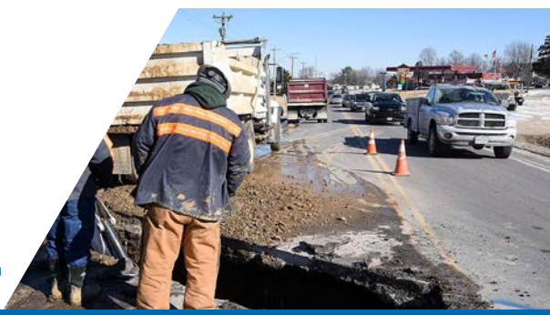
Extreme winter weather leads to city water line problems under 28. See page 8.
