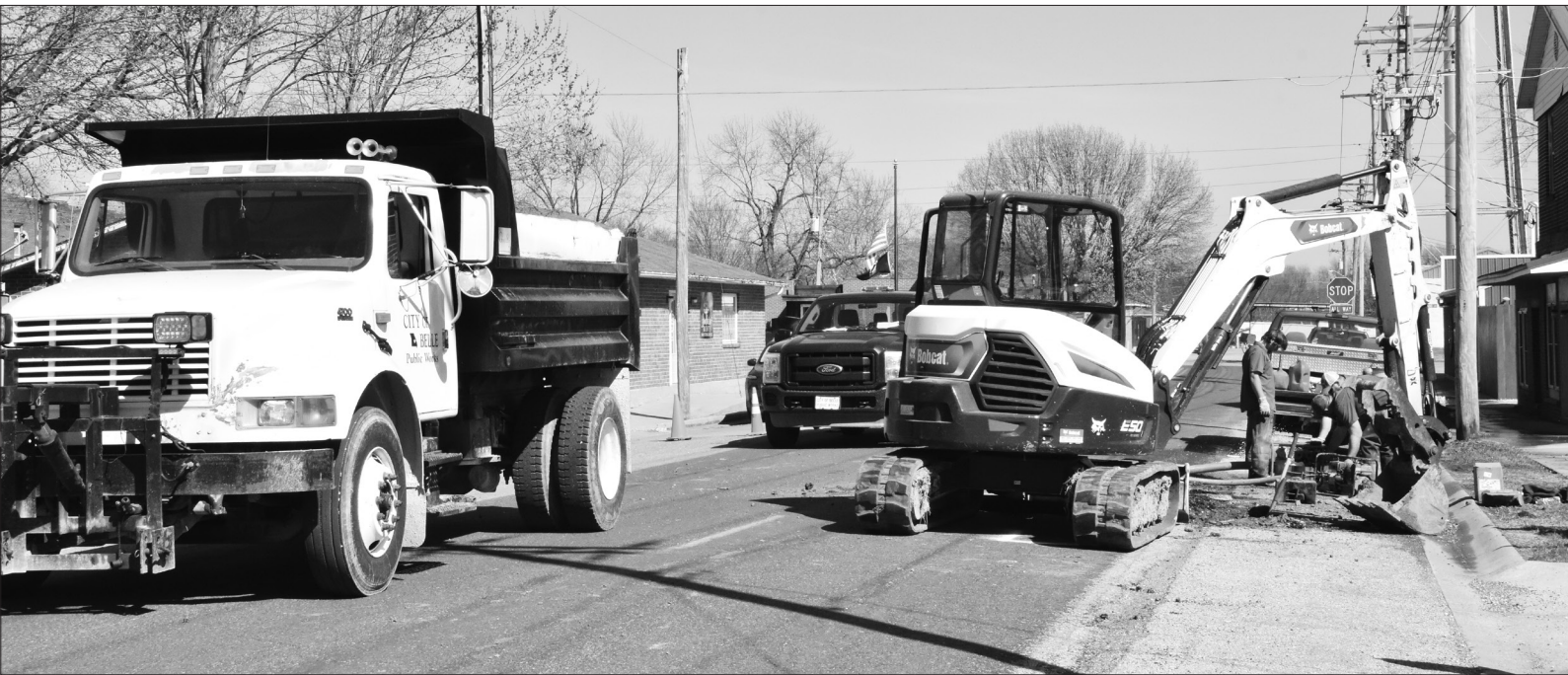
BELLE PUBLIC Works employees on March 20 were called to a water main break on the corner of Third Street and Alvarado Avenue. What started as a small leak turned into a big problem. The pipeline, estimated to be about 100 years old, disintegrated when employees attempted repairs. The pipe burst and left many residents without water.
