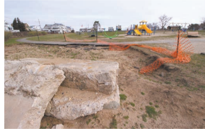
STILL WAITING: Work started but then stopped in the fall on the site for adult exercise equipment at the Conimicut playground. It is to resume shortly say Parks and Recreation Director Bev Wiley.
